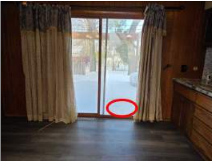
The glass was cracked in this door.
