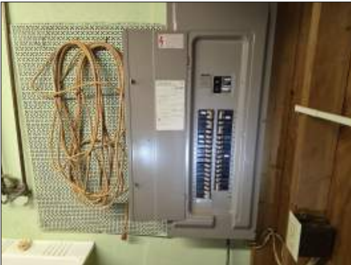
This is the main electrical panel.
