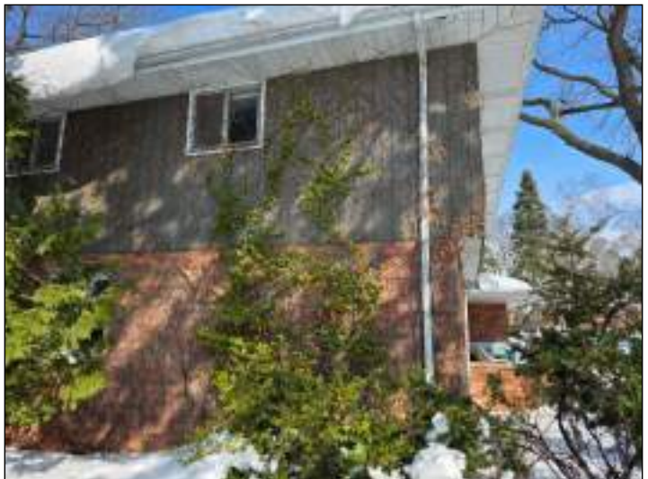
I recommend removing the vines.
