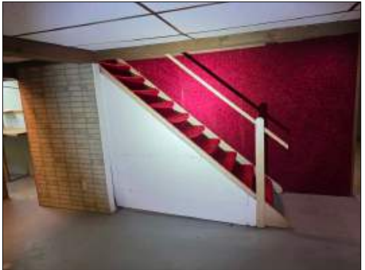
I recommend adding a guardrail on this stairway.
