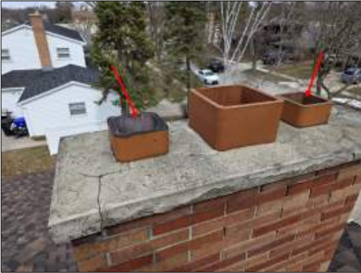
I recommend capping off these two unused flue pipes.
