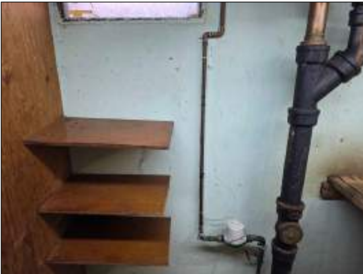
Some small cracks were observed in the foundation.
