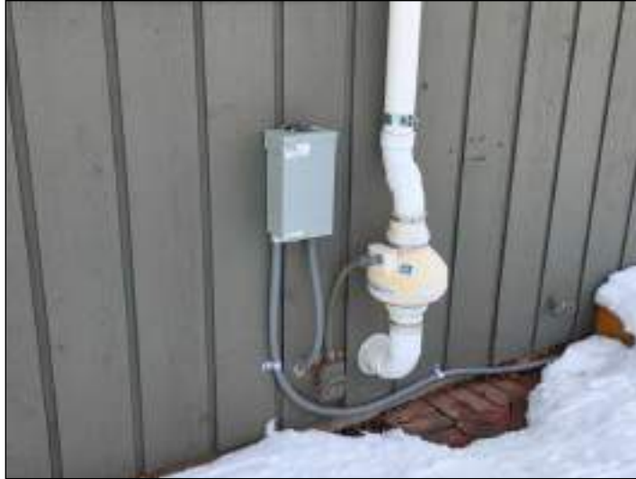
A radon mitigation system was installed on the exterior of the house.
