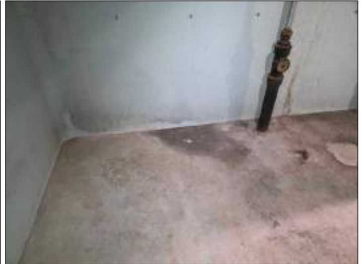
Some old moisture stains were observed along the foundation walls.
