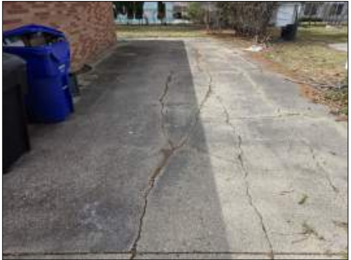
The slabs were heavily cracked in this area.
