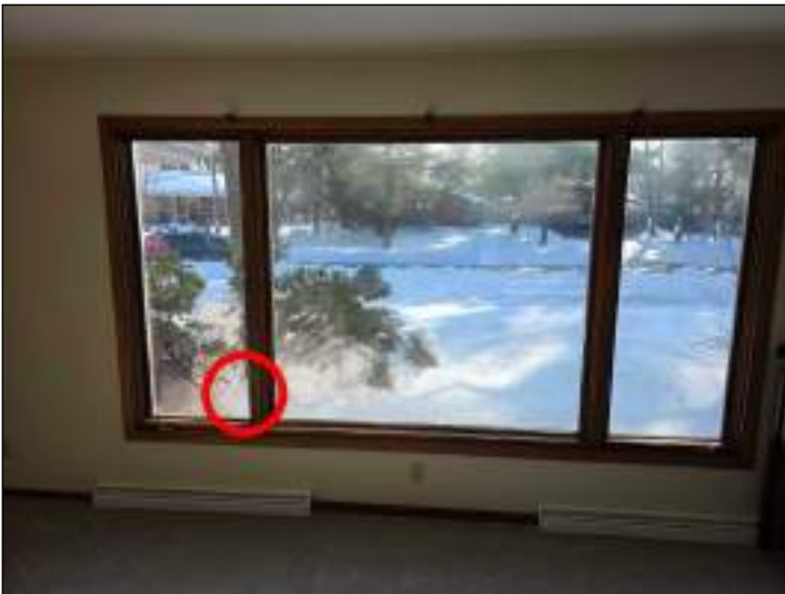
The lock lever was damaged on this living room window.
