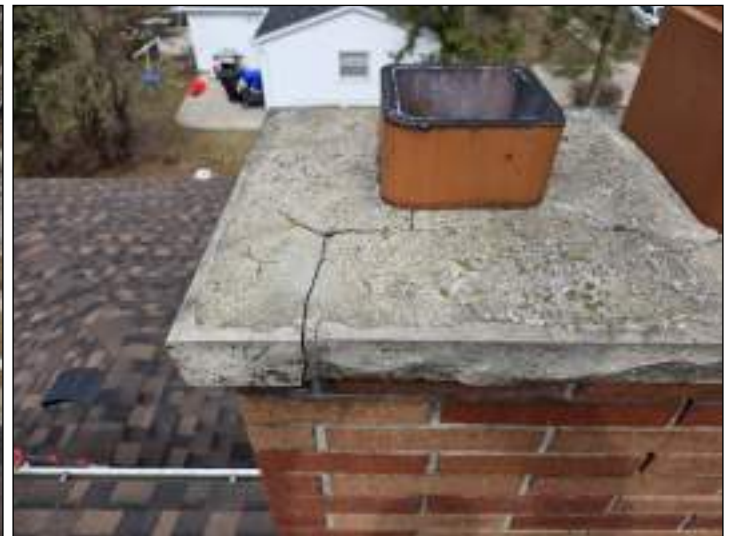
The crown was cracked in a few areas.
