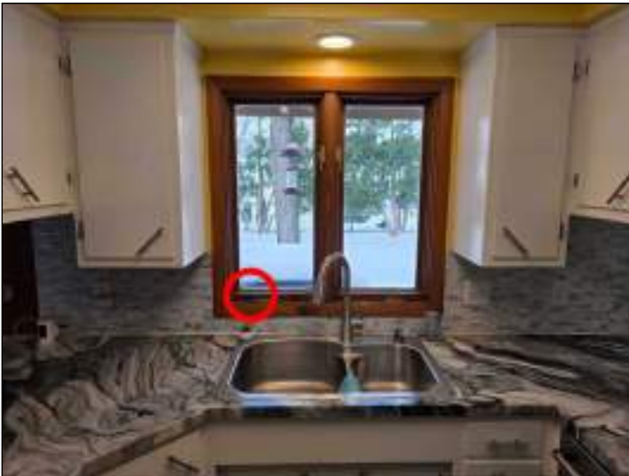
This kitchen window had a stripped crank mechanism.
