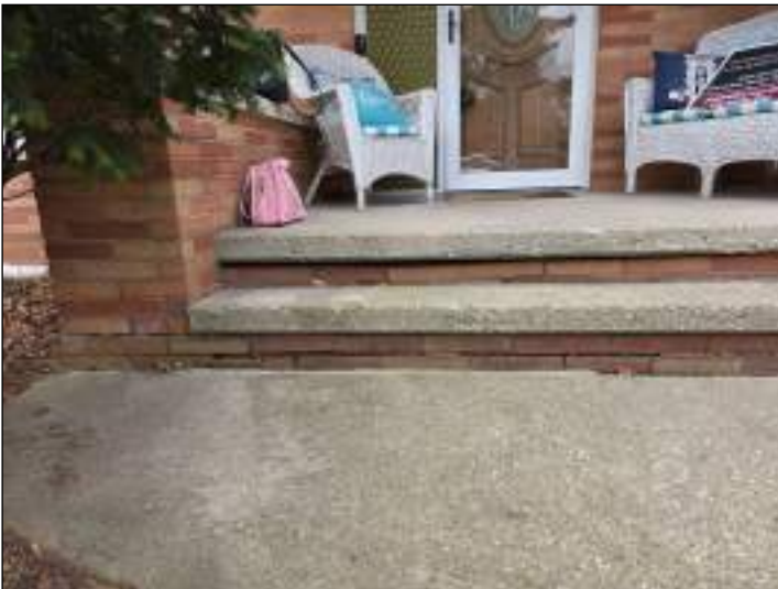
The mortar was cracked or missing in some areas.
