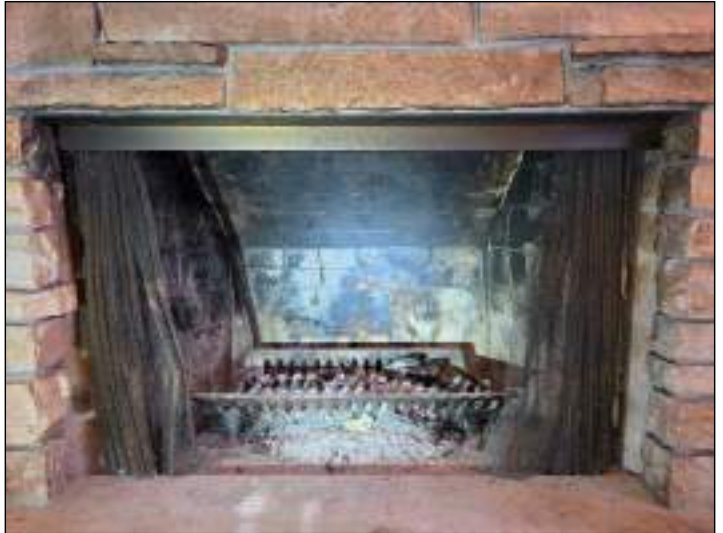
Some of the bricks in the firebox were cracked.
