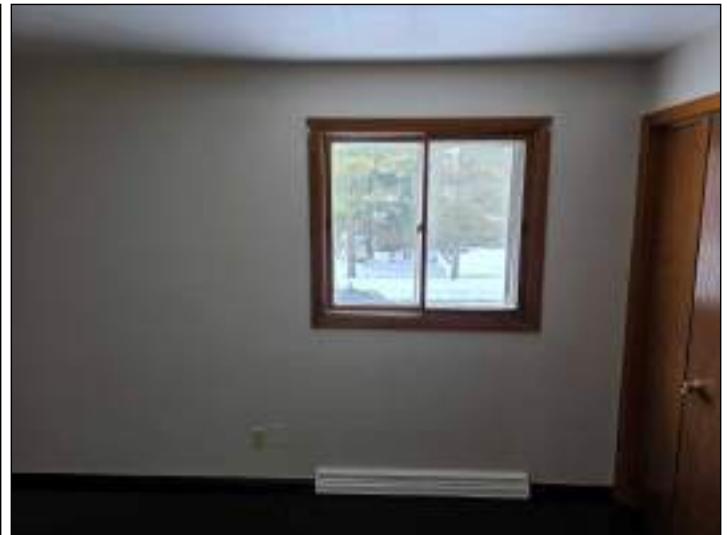
The northeast bedroom window had a damaged storm window, and the slider window was loose from the frame.
