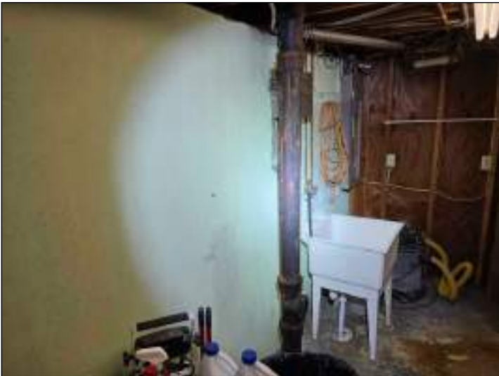
Rust blisters were observed on the cast iron pipes.
