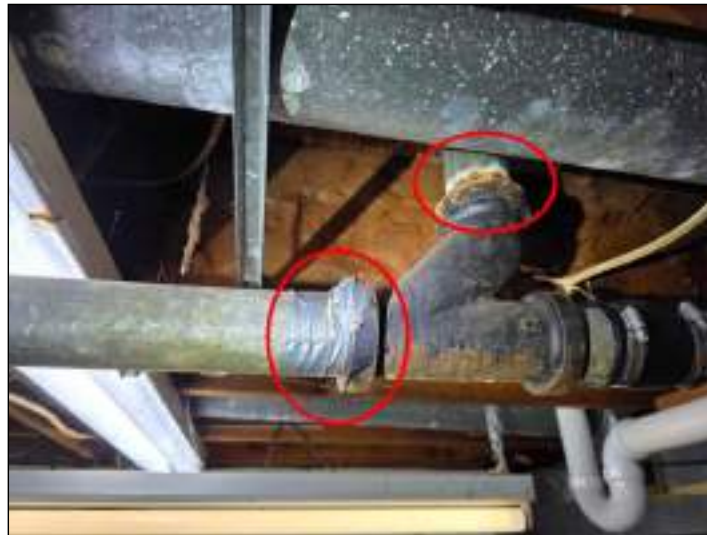
The drain pipes were rusting in several areas.
