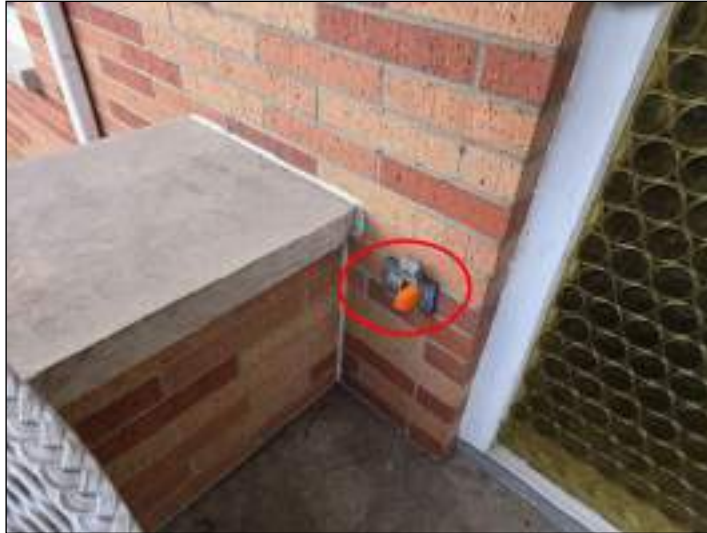
GFCI protection was missing on this outlet.
