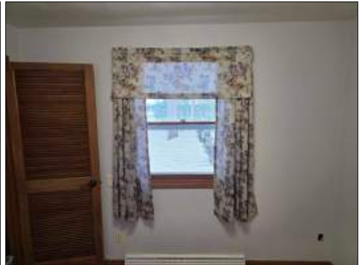
The glass was loose in this first-floor bedroom window.
