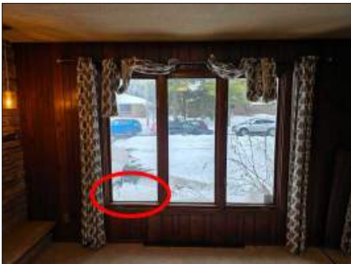
This family room window rubbed on the frame making it difficult to close.
