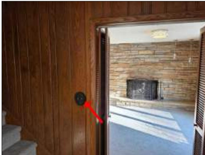
This three-way switch was miss-wired.
