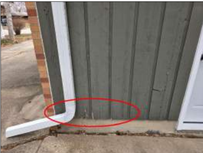
The siding was starting to rot along the bottom of this wall.
