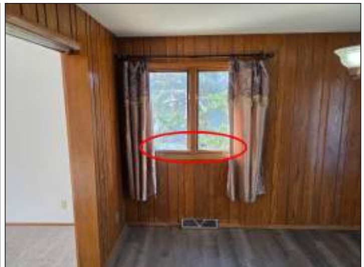
Both of these dining room windows rubbed on the frame, making them difficult to close.
